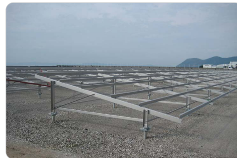
Solar panels supporting frames made of Duplex Grade SUS821L1 Picture Courtesy NIPPON STEEL Stainless Steel Corporation
