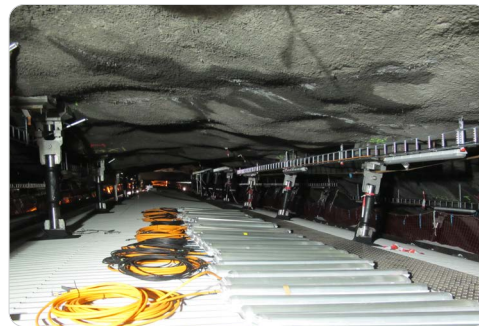
Dynamic hangers in Holmestrand train tunnel Picture courtesy of Sandvik Materials Technology
