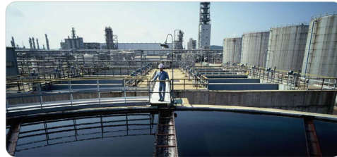
Waste water treatment plant Picture courtesy of Institut de la Corrosion
